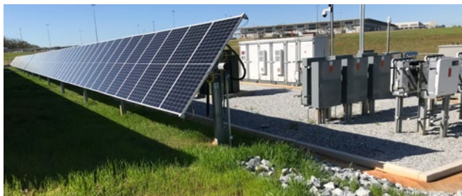
Utility-scale storage technologies are helping electric co-ops improve reliability, integrate renewable energy and manage infrastructure costs.
